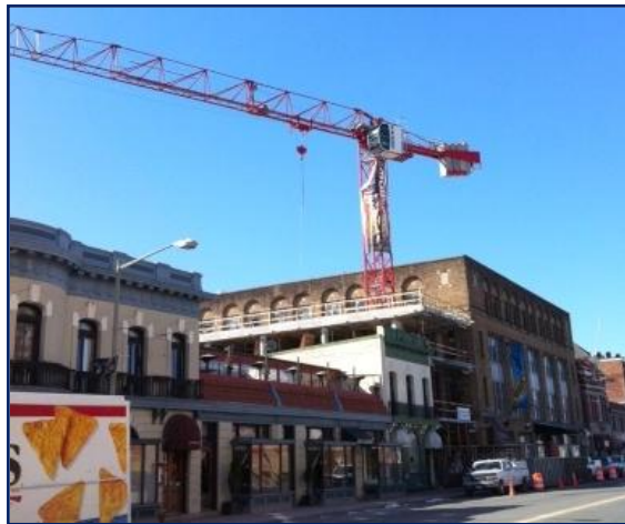
Figure 5: Tower Crane Located in Center of New Addition, Picture Courtesy of Luis Ortiz
