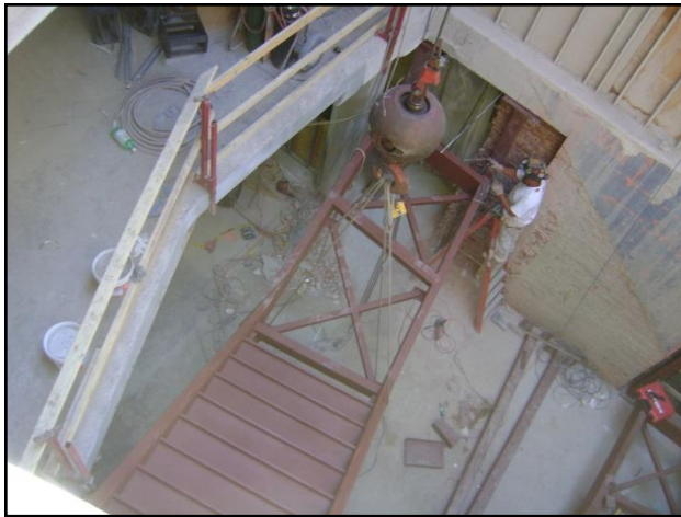
Figure 1: Stair Section Suspended by Crane through Slab Cut; Picture Taken by Clara Watson
